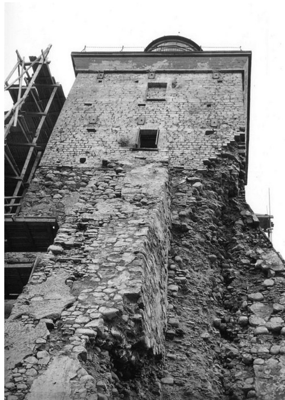
The damaged Kõpu Lighthouse surrounded by scaffolding in 1988, Hiiumaa Museums Foundation.
