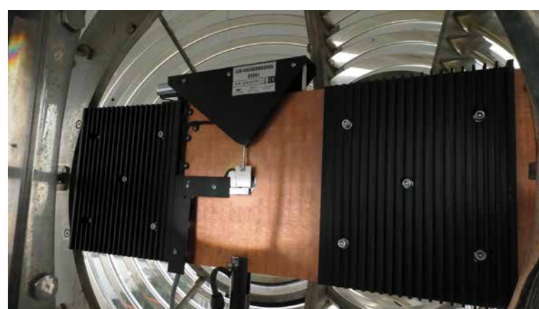
In 2020, a Sabik E8201 LED lantern fitted with heat sinks was installed inside the Fresnel lens of the existing optical apparatus, photograph by T. Rosenberg.
